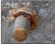
Corroded VA screw in aluminium
