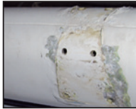
Corroded aluminium mast
